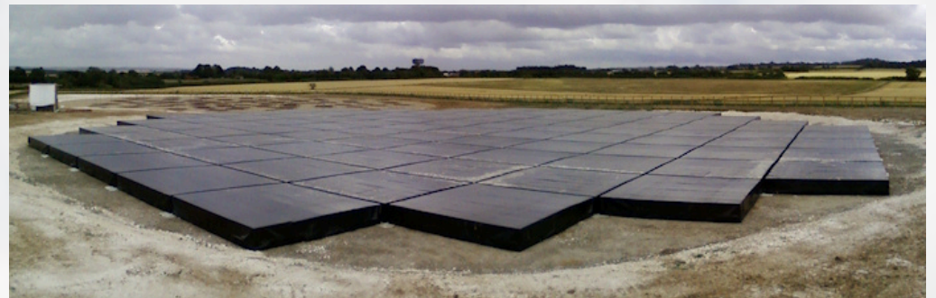
LOFAR-UK Chilbolton, High-Band Array 120-250 MHz comprising 96 tiles x 16 cells x 2 directions = 3072 elements.
